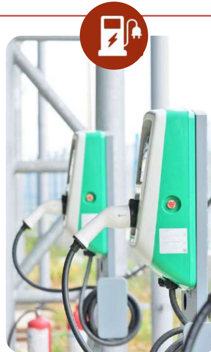
Electric vehicle charging stations
